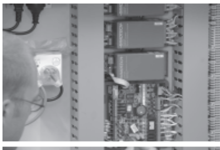
John Collins of the AAT's Electronics Section working on the air handling control system of the AAT Dome air conditioning. Photos Jonathan Pogson
